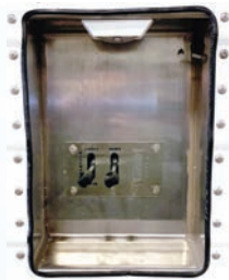
Conveyor control panel with light
